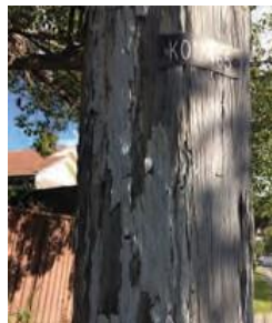
Asbestos containing paint
