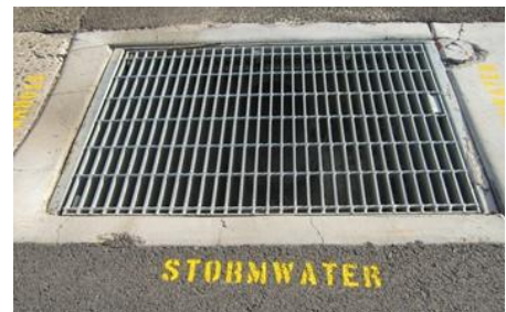
Check whether nearby drains go to stormwater, sewer or the oil containment tank
