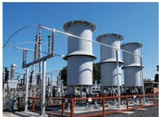
Air cored reactors
