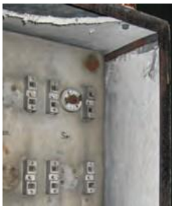
Millboard lining inside the fuse box
