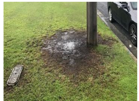
Contamination from a leaking pole transformer
