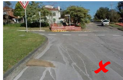
Saw-cutting slurry has not been contained effectively
