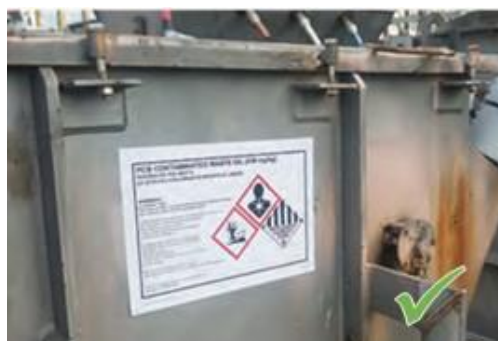
PCB waste labelled ready for collection
