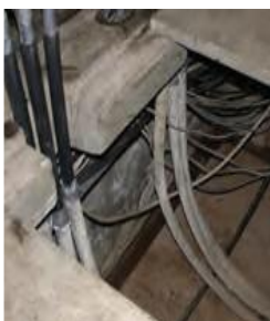
Feeder cables at zone substation
