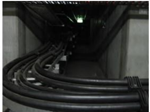
Cable terminations and pits
