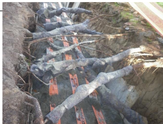
Where roots are exposed for extended periods of time (>24 hours), wrap larger roots (> 50mm diameter) in jute mesh or hessian and keep moist
