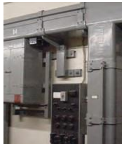
Busbar trunking and fuse box
