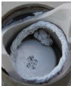
Moulded cement Asbestos rope inside broken fuse
