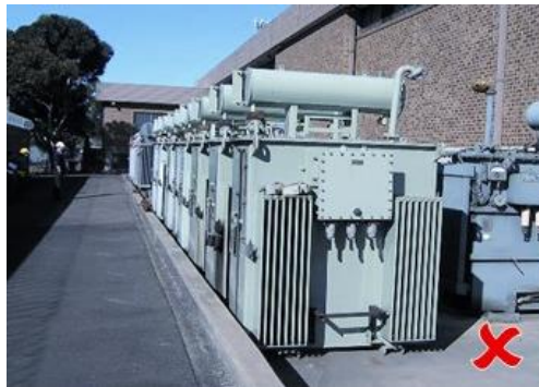
Equipment stored too close to the bund wall means leaks may not be contained
