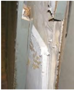
Damaged fire door exposing asbestos core
