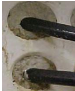
Non-chalking compound in substation wall
