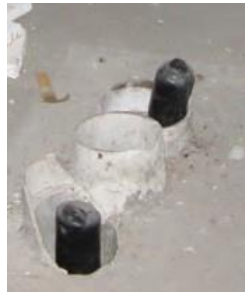
Conduits in substation concrete floor
