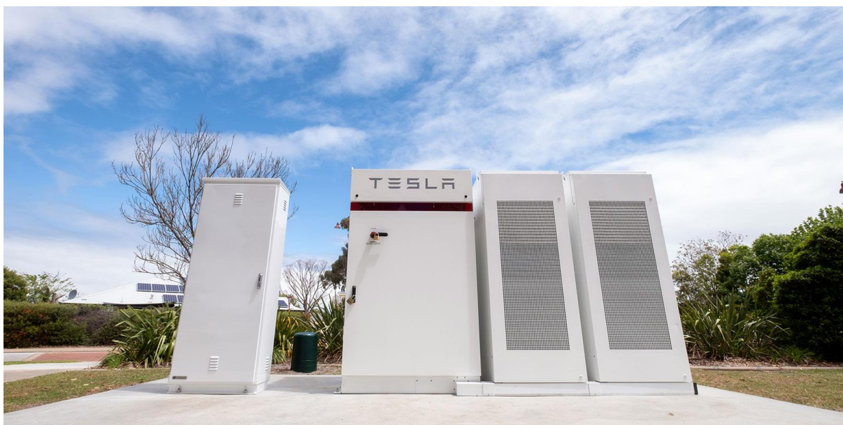
Figure 6: Western Power Community Battery
